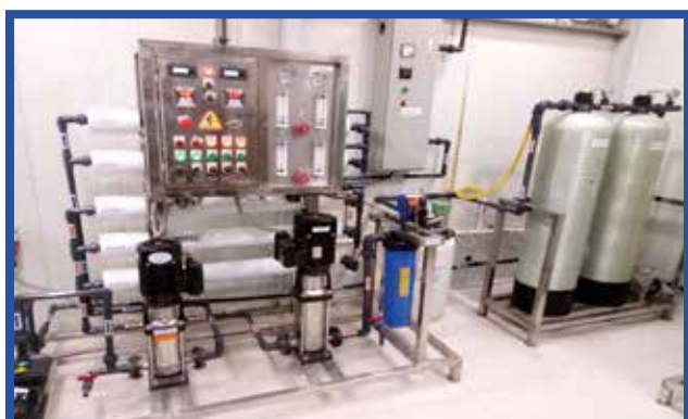
Double Pass RO Water Plant (All Size Capacity)
